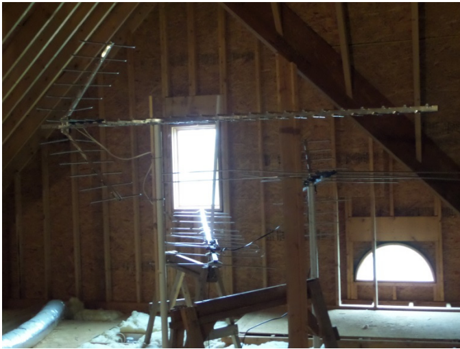
Top Foreground = Channel 16 UHF Deep Fringe Antenna Aimed at Whitehall SC Bottom Left = VHF Yagi Aimed at Savannah
